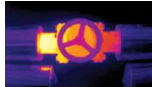
Thermal camera view of the uninsulated valve
